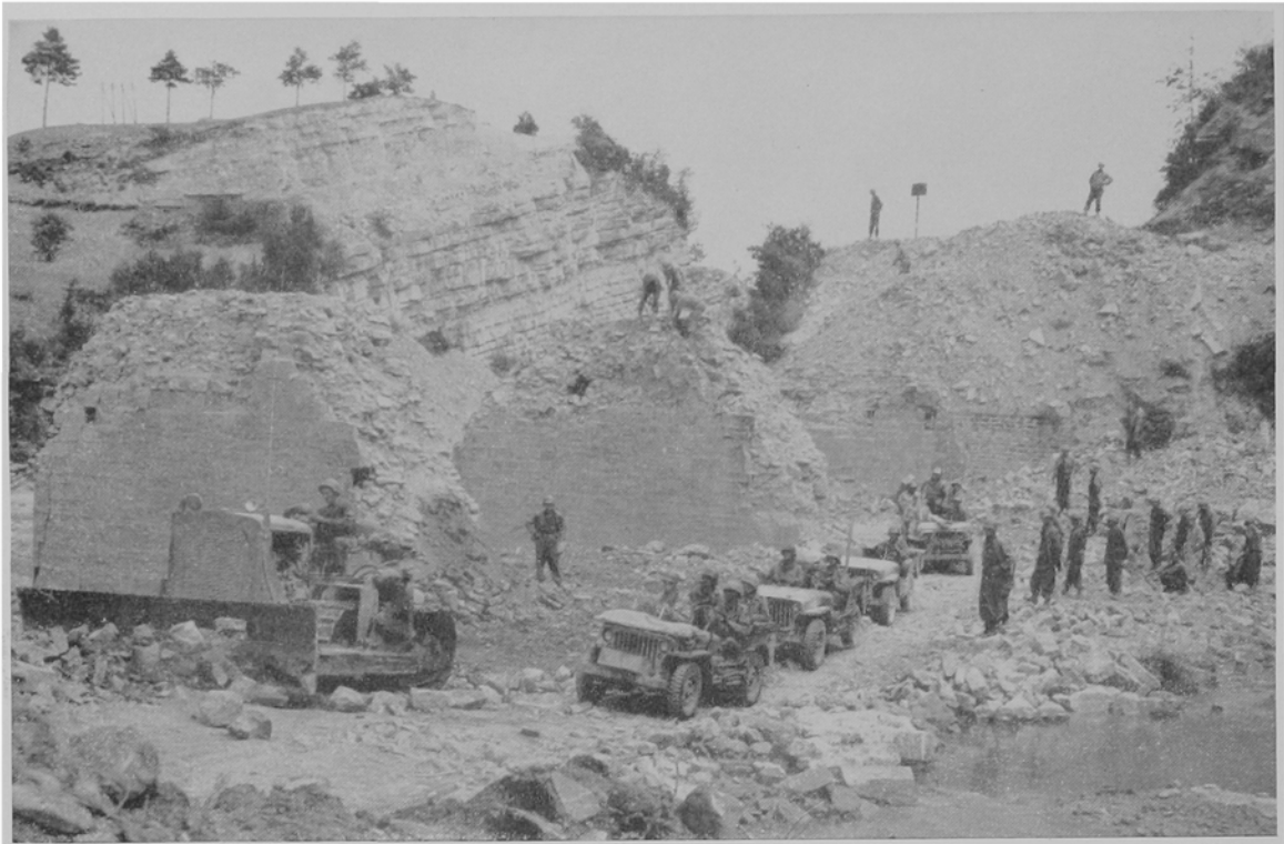
Jeeps wait for a bulldozer operator to complete a bypass near Firenzuola
